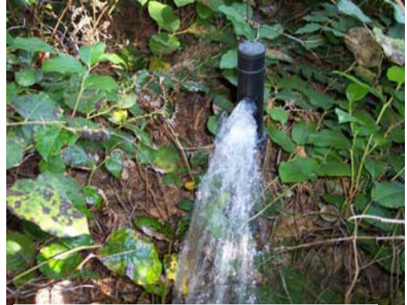
Leaks can be costly! Repair leaks promptly. 1
